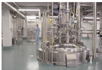
The top of a reactor vessel at the Indena plant.
